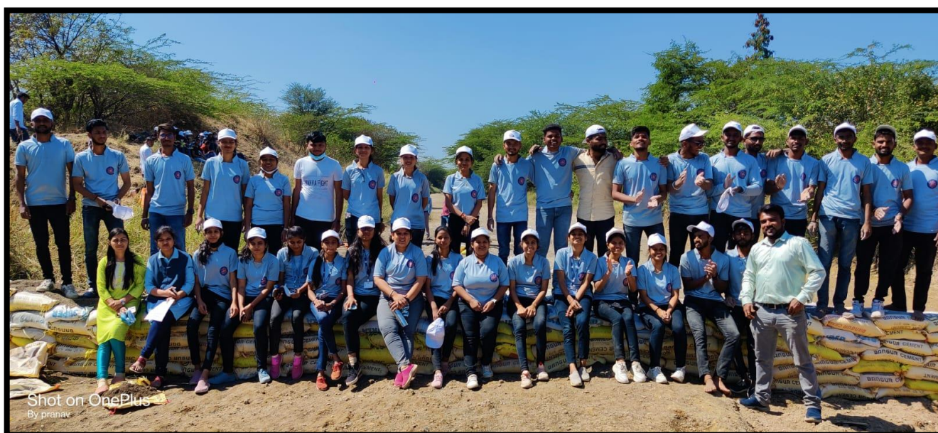
NSS volunteers construct a 30 ft. long , 5 ft High and 6 ft wide damp / embankment at Village Khadki
